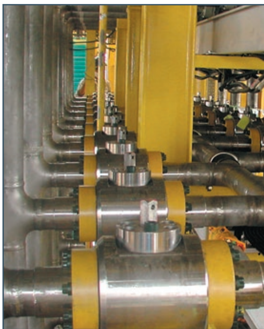
Manifold assembly prepared for actuator installation.
