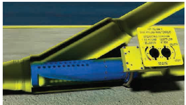
Director Sleeve rotated Permitting Bi-directional Pigging in Mainline
